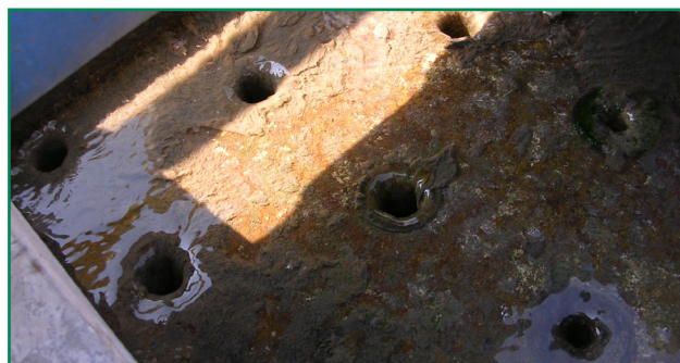
Highly fouled cooling tower basin.
